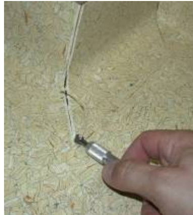
Grooving is necessary to weld angles and corners in a watertight and GMP compliant manner.
