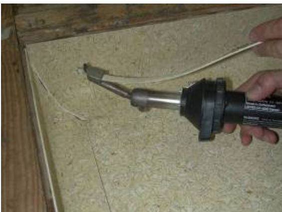
With a small hot air gun and the appropriate flat welding nozzle...
