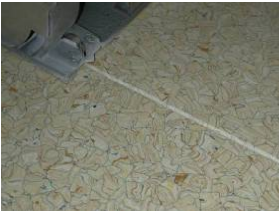
Finally, groove and weld the junction lines between skirtings and floor tiles.
