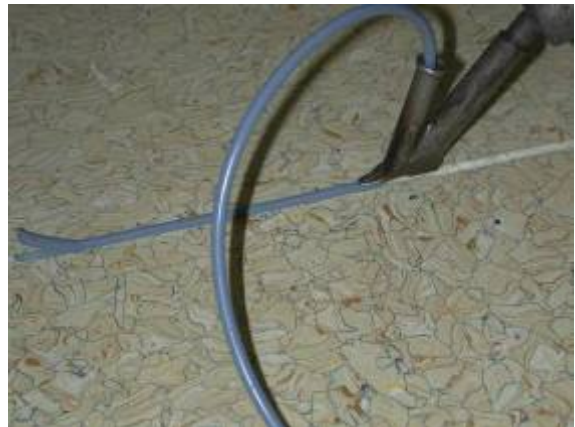
This welding is close to the wall and welding by hand might be necessary
