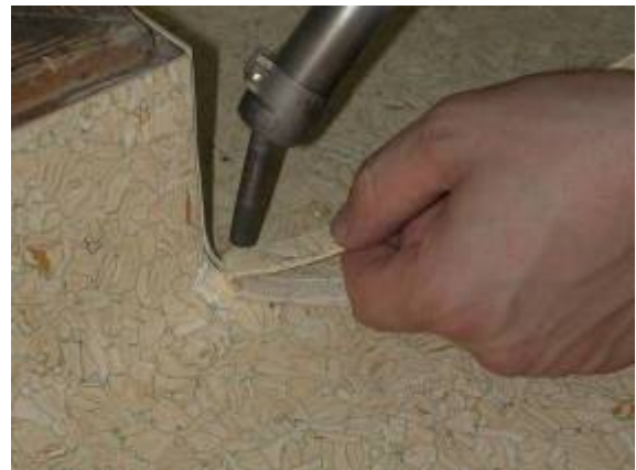
Weld outer corners as shown: Start welding the stripe at the beginning of the cove...
