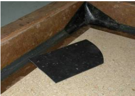
Skirting need a rounded end to fit in the coved corner. To prepare a template as shown, make a drawing by pressing a sheet of paper on the coved corner and following the curve with a pen.
